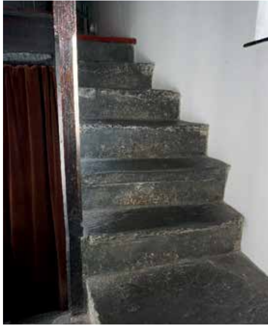
And dangerous stairs
